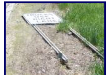
Figure 6. Typical Roadside Signage
