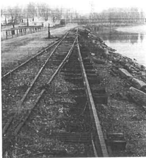
Photo B2: View of the dike crest looking towards the right abutment.
