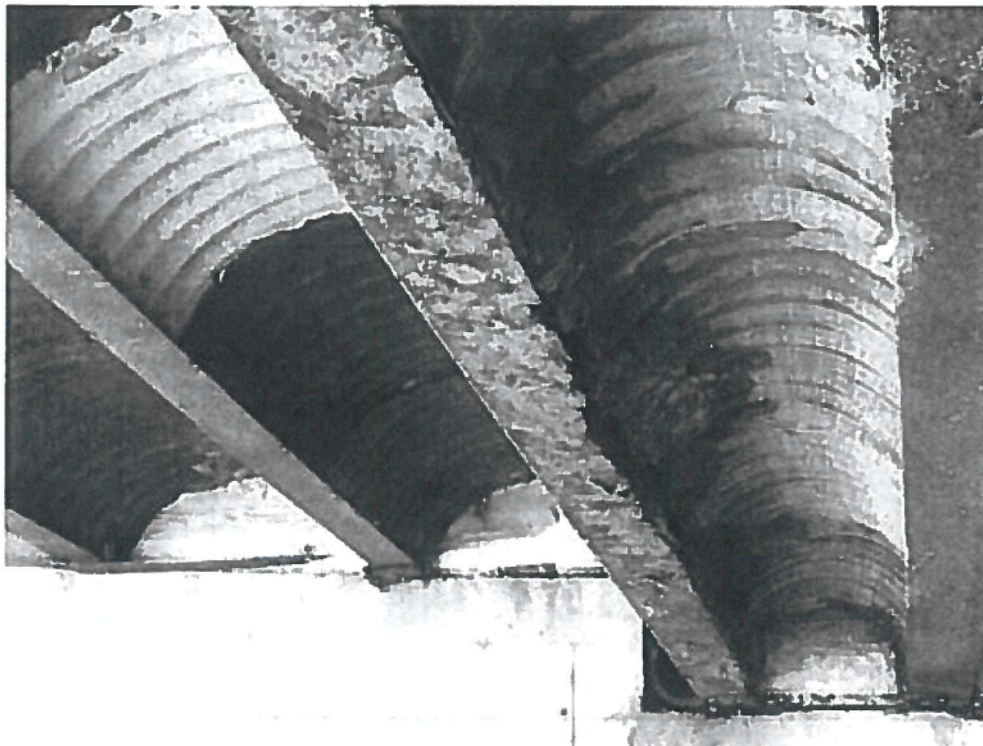
Photo 4: West edge of the bottom flange of beam #25.
